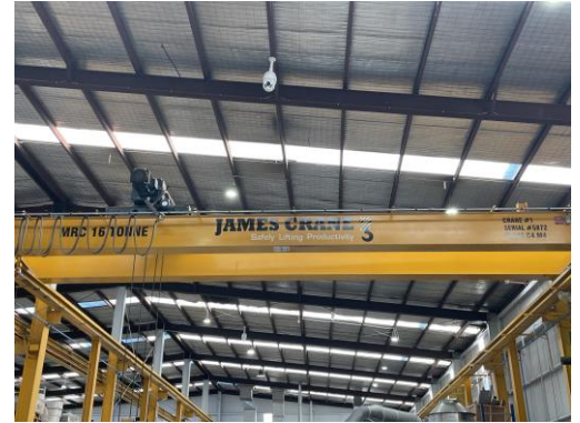
16 Tonne Overhead Crane
